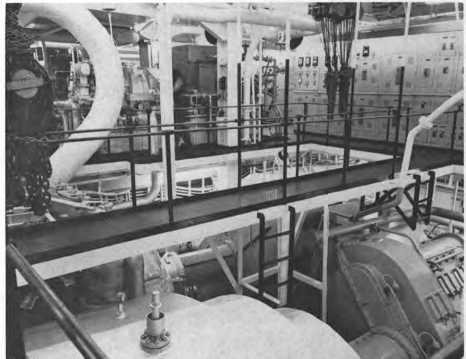
Auxiliary machinery is located on the well lighted upper engine room level.
