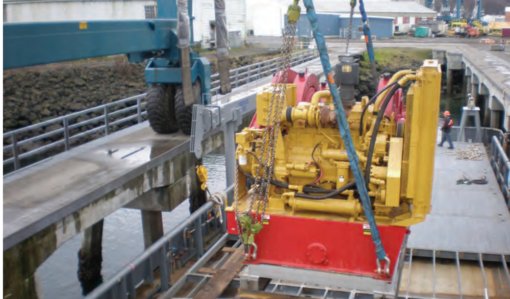
A Manitowoc 390 winch being lifted aboard the Quest in Port Angeles, WA
