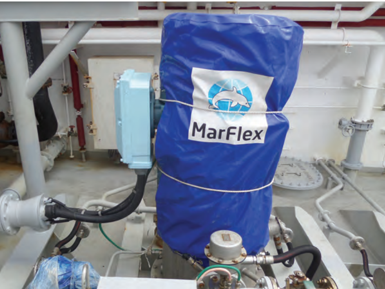
Marflex Variable Frequency Drive Cargo pump.
