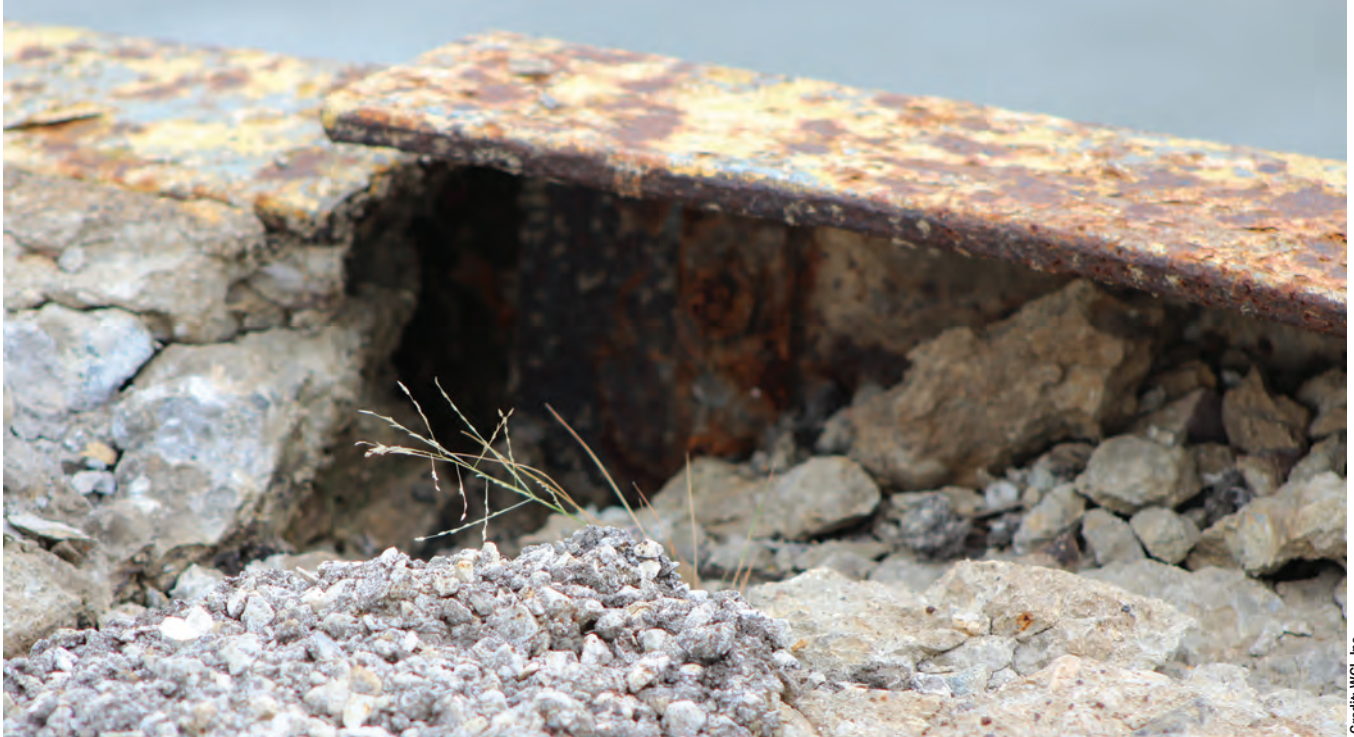
Severe deterioration of infrastructure at the Lagrange Lock and Dam in Illinois.
