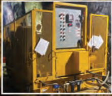
SHAFT SINKING WINCHES
