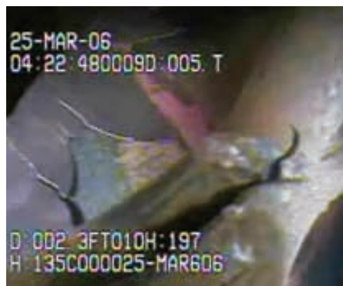
A cracked seam.
