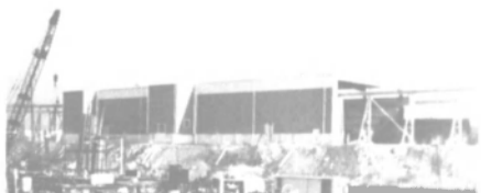
A new steel-plate fabrication shop is now forming steel plate up to 1/2 inch thick and up to 41 feet long at the National Marine Service shipyard at Hartford, Ill.
