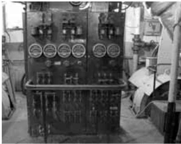
OSHA, where were you when we really needed you? 1931-vintage electrical control panel is one of two in Harvey's engine room, this one to control the pumps. It says "Danger" twice. A larger one aft controls the propulsion motors, and has even more of Dr. Frankenstein's exposed switches. (Photo: Don Sutherland)
