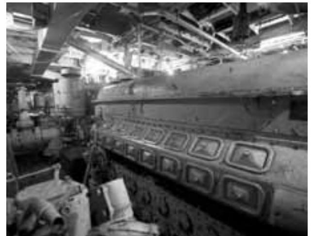
The Harvey's broad engine room is packed with machinery, including five main diesels and two auxiliaries, pumps, and much unique equipment. The owners recently bought two Fairbanks-Morse OPs for parts, and welcome contributions of equipment and supplies. (Photo: Don Sutherland)
