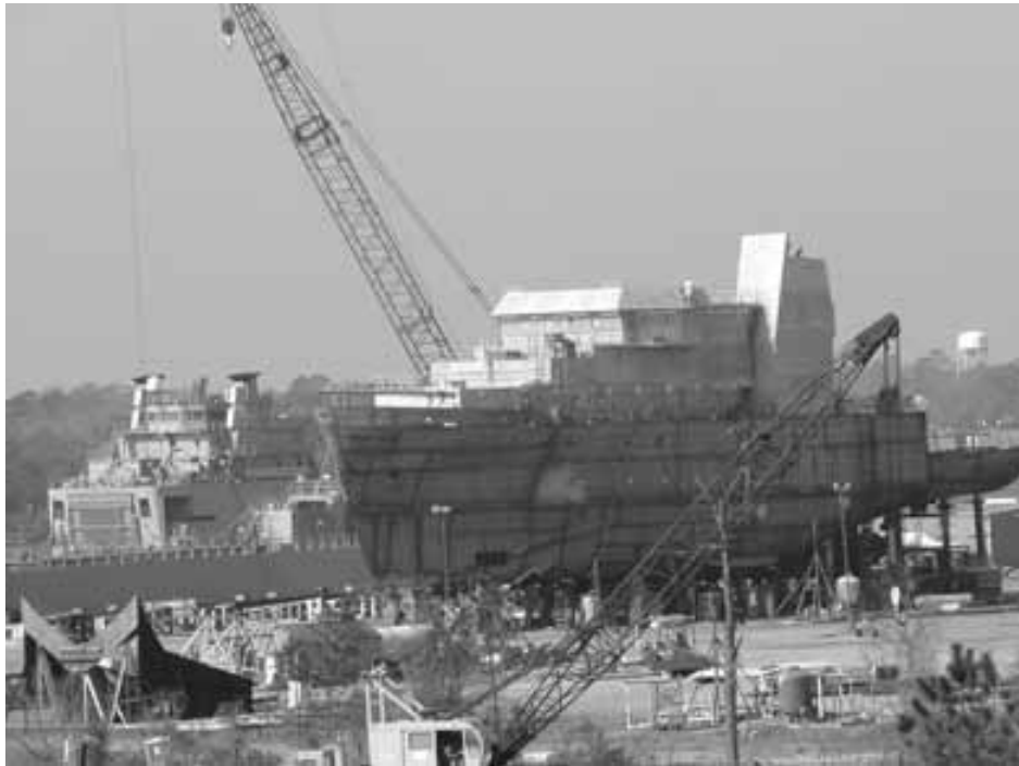
The Henry B. Bigelow under construction on land at a VT Halter Marine shipyard.
