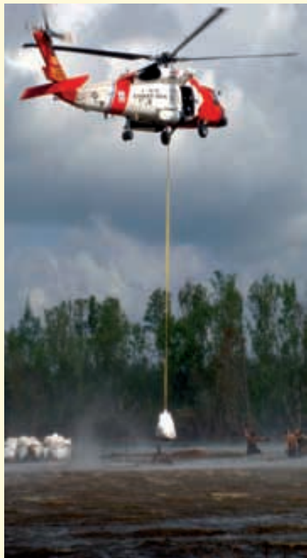
A Coast Guard HH-60 Jayhawk helicopter crew from Kodiak, Alaska, based out of Air Station Houston drops a sandbag to repair a damaged levee. The Coast Guard dropped more than 700,000 pounds of sand while working hand in hand with the National Guard to reconstruct the breached levees. U.S. Coast Guard photo by Christopher Evanson
