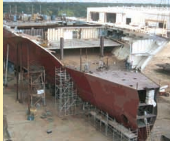
This August 2003 photo shows the state of completion on the Jean Anne a few months after work restarted in February 2003. (Photo Credit VT Halter Marine)
