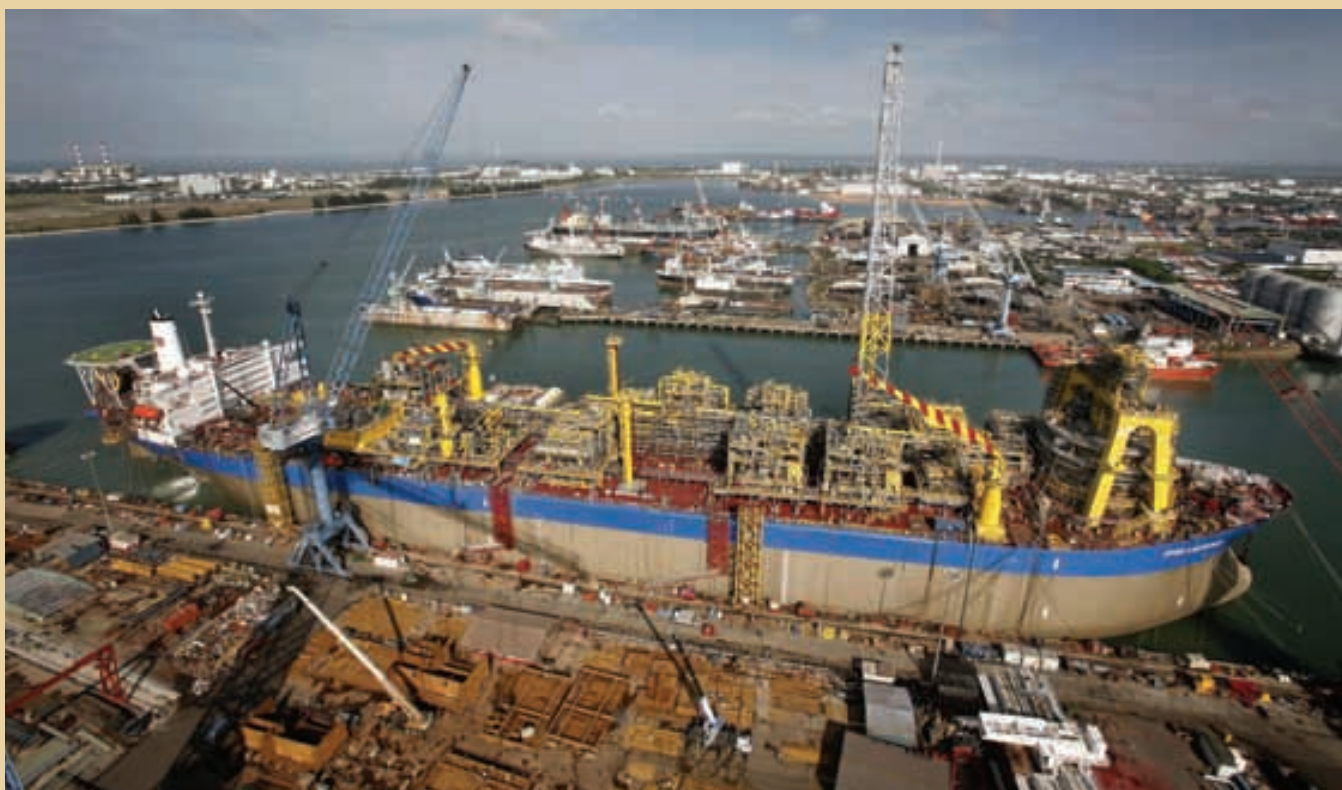
Keppel Shipyard successfully completed the sixth Floating Production Storage Offloading (FPSO) conversion project from SBM since 2000.
