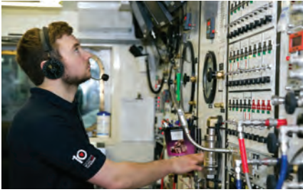
Sat control room onboard a Bibby OSV.
