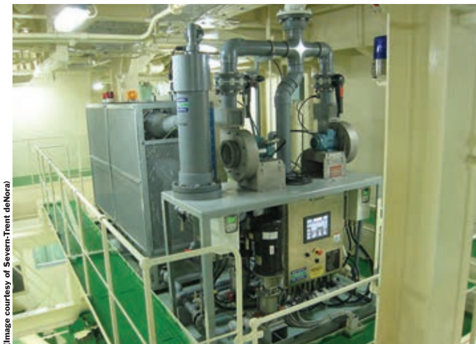
Shipboard installation of electrochlorination system for generating sodium hypochlorite.
