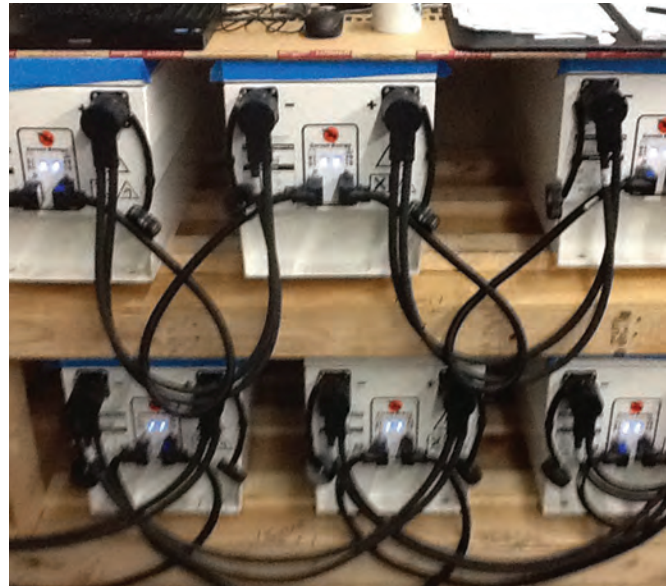
Corvus lithium batteries in operation during hybrid engine testing at Northern Lights facility Seattle, Wash.
