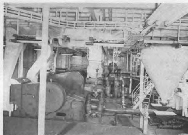
Pump room with mixing pump and mud pumps behind it.
