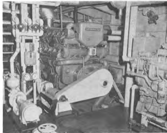
One of the engines equipped with Blount fire-pump drive.
