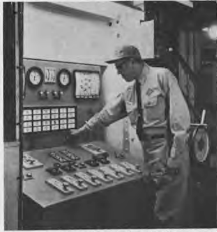
Figure 1—The Cadillac's chief engineer, C.R. Mihalick, shown at the engineer's console, located on the engine control level.
