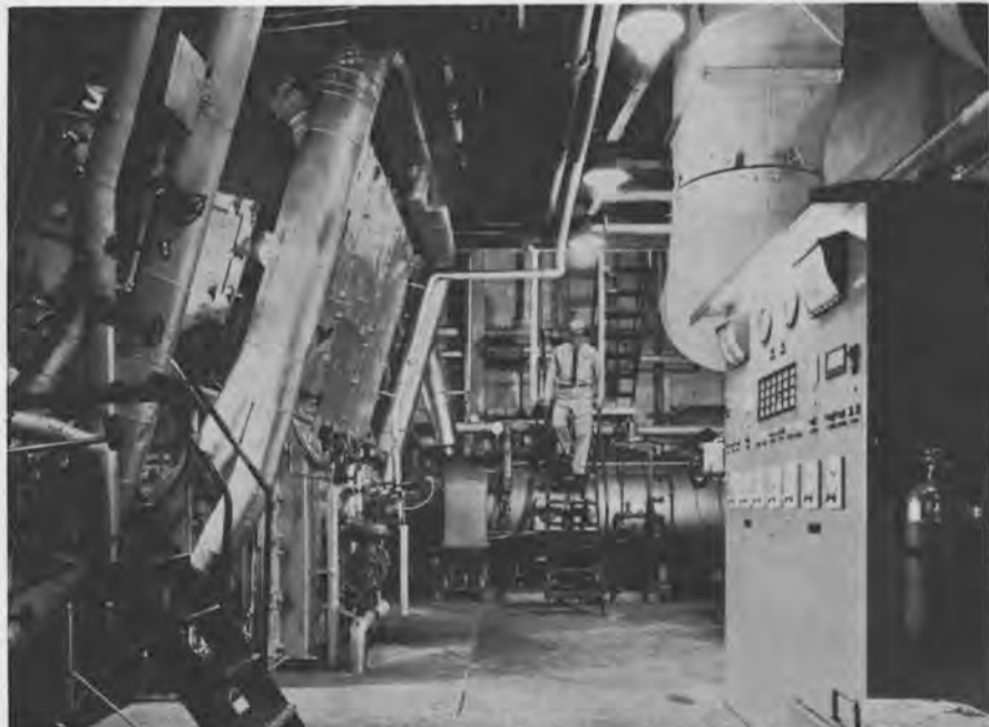
Figure 2—The boiler room on the Cliffs vessel, Cadillac, is normally unattended. The panel at the right duplicates the controls on the engineer's console. These controls are normally used only during initial boiler start-up. The boiler fronts are at the left. These contain Bailey FLAMON Flame Detectors, ignitors, and B&W burners. Beneath the stairs (center) is a horizontal donkey boiler that provides heat when the vessel is in port.
