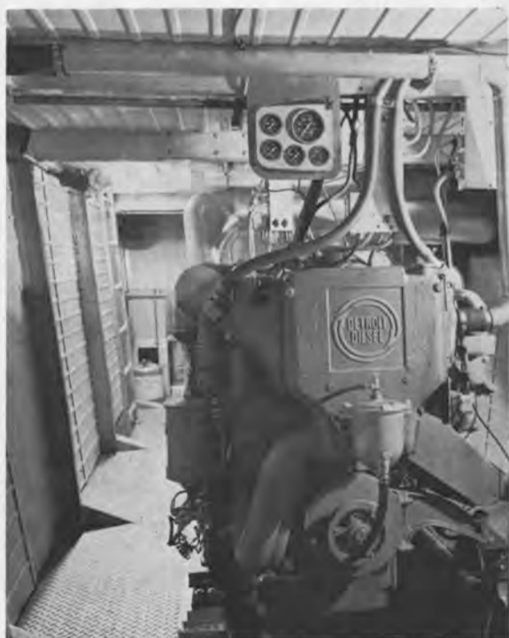
Looking aft in starboard engine room showing turbocharged 12V-71 Detroit Diesel main engine. Also visible in the photograph are the engine room exhaust blower, hydraulic reservoir and fixed CO 2 extinguisher system.
