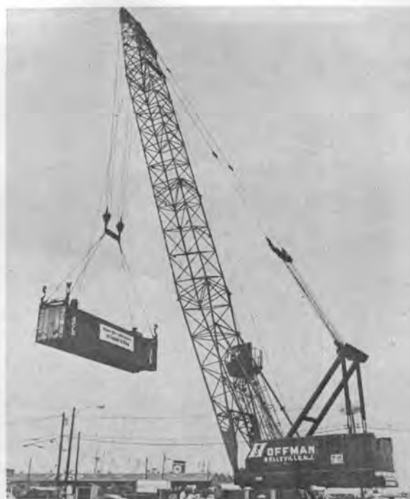
The largest mobile truck crane in the United States demonstrating its unique container-handling capability. An elevated cab and a special container tip enables easy leveling of an unbalanced container and the automatic container spreader frame. This machine represents Hoffman Rigging Service's latest and most modern container-handling mobile crane.
