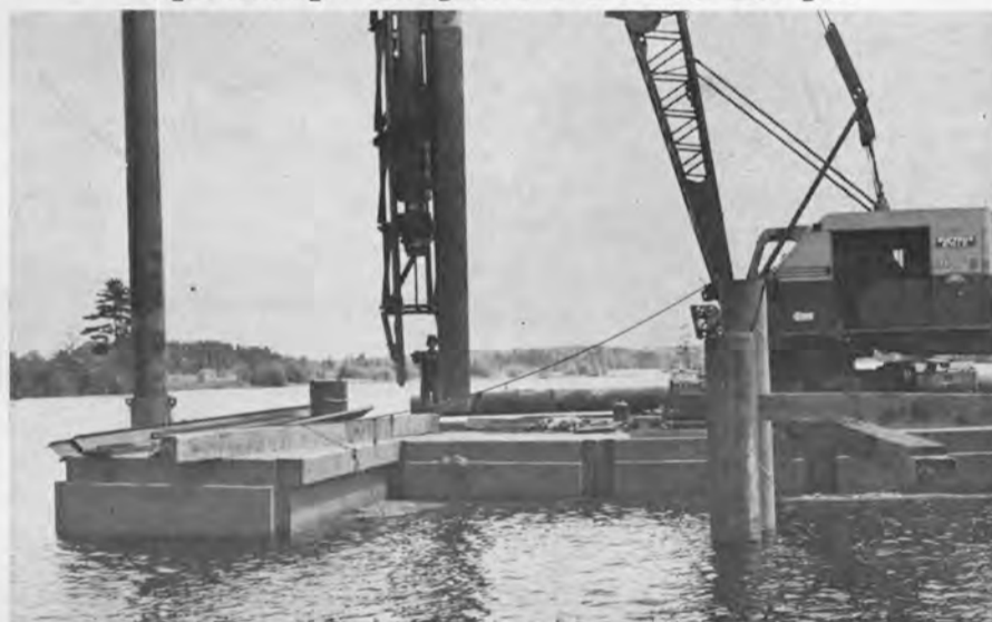
PORTABARGES being used to support a pile driver. This view shows the patented method of interlocking the barges and the variety of shapes that can be formed.
