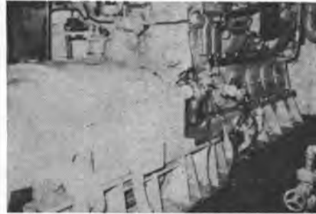
DIESEL GENERATOR SET
