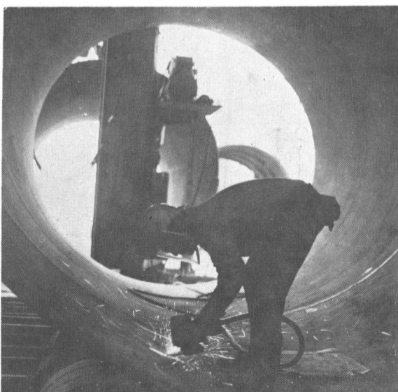
Grinding Operation —This worker is shown as he smooths out the steel in a tubular section of a semisubmersible mobile offshore drilling platform. Marathon currently has an employment of 1,800 in the new yard.
