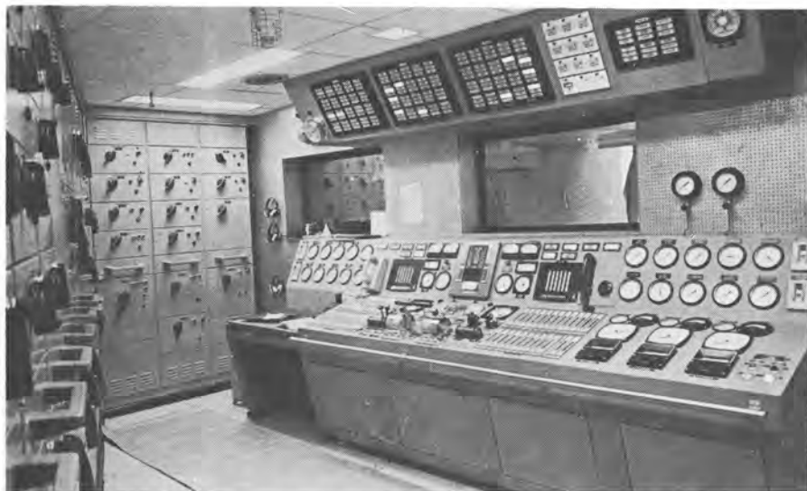
The consoles shown here in the engine-room control station were designed and built by the shipyard. The windows provide a view of the engine room.
