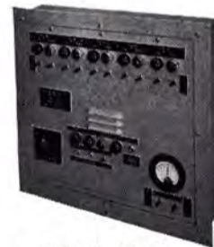
FIRE AND GENERAL ALARM PANELS
