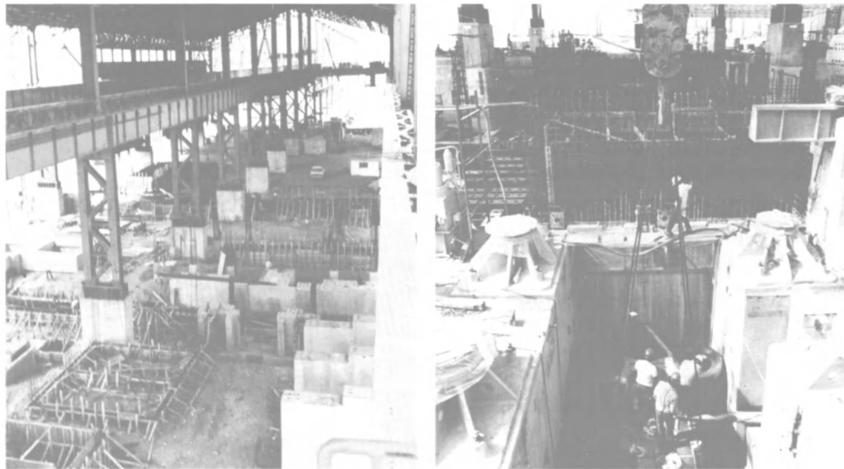
Interior of the steel making shop under construction at the NKS facility.
