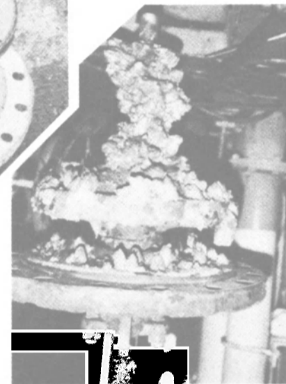
After 17 months of C 2000 operation the same sea valve at inspection
