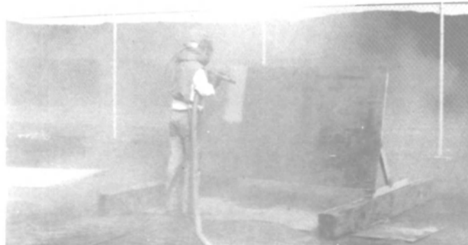
Dust (shown here from silica sand) means lower cutting efficiency and visibility and increased health hazards and clean-up costs.
