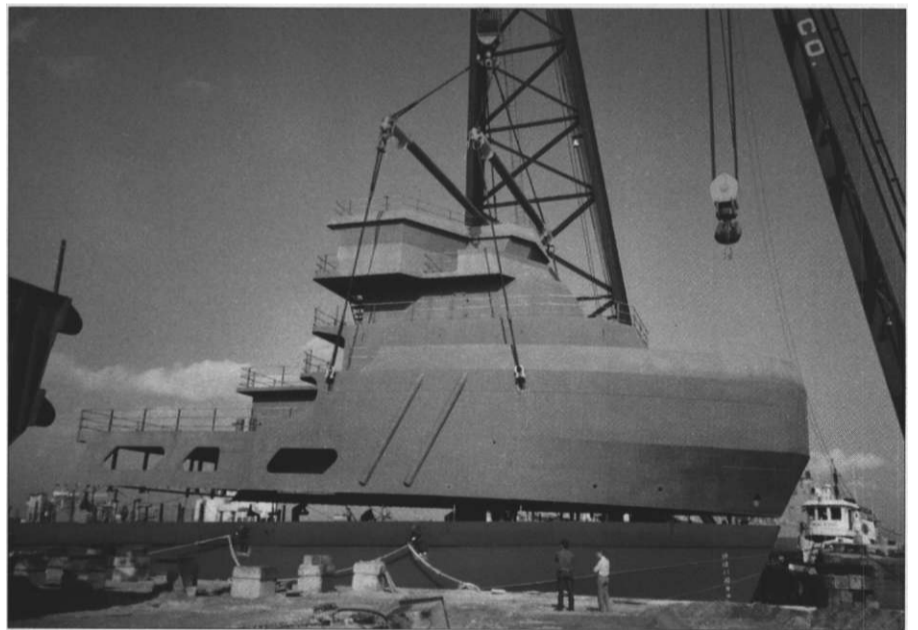
The 200-ton superstructure of the Gulf Responder being lowered into place by the 600-ton derrick barge Lili Bisso at the Mobile shipyard of Bender Shipbuilding & Repair Co., Inc.
