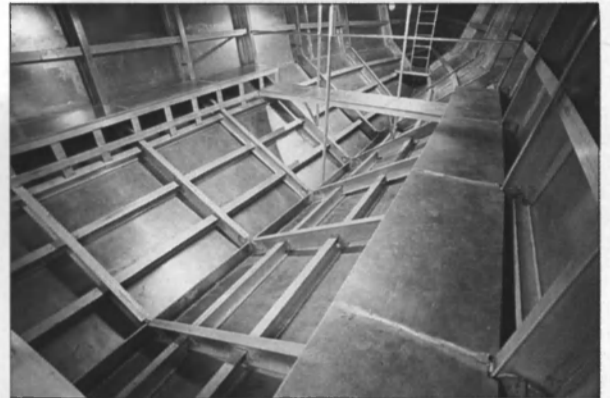
Hull interior of the Global I, built using Falcon Maritime Ventures' patented aluminum construction process.
