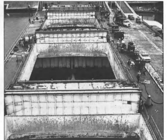
The four corrugated cargo bulkheads of the self-unloading bulk gypsum carrier, M.V. Georgia-S, were completely replaced by the General Ship Repair Corp. in Baltimore.
