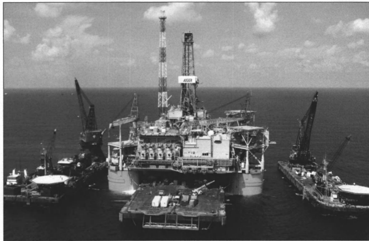
Pictured: McDermott's Derrick Barges 16 and 28 were moored adjacent to the hull and provided crane and rigging support and quartering for mating operations. McDermott's Derrick Barge 50 was used to install the preset portion of the lateral mooring system.
