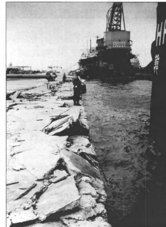
Damage to the quay resulting from contact with the OHI 5000 . Typhoon Seth also resulted in the grounding of five smaller crane barges in the area near Ulsan, South Korea.
