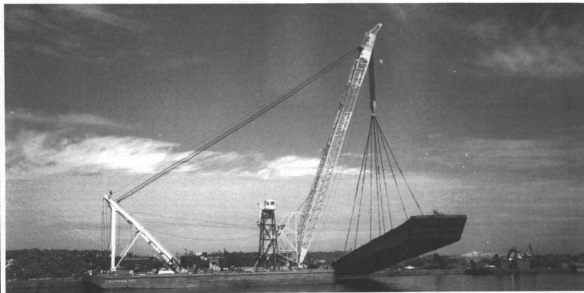
Derrick Barge CHESAPEAKE 1000
