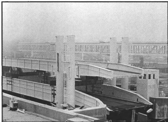
The RoRo facility for ferry terminal I at Puttgaden is shown during construction.
