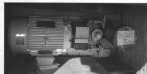
15 Foam Fire-Fighting Pumps Mfg: Blackmer 35GPM@200psi Horizontal Model BXL1/25NFC-TB Motor: Reliance 7.5HP 440/3'60 With Controller, Spares and Educator Assembly
