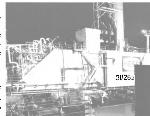
Verolme Botlek placed a new 80-ton hull section into FPSO Uisge Gorm at its Rotterdam yard.
