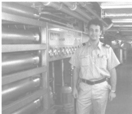
Zuiderdam's environmental officer, Willem Berends provided a tour of the engine room.
