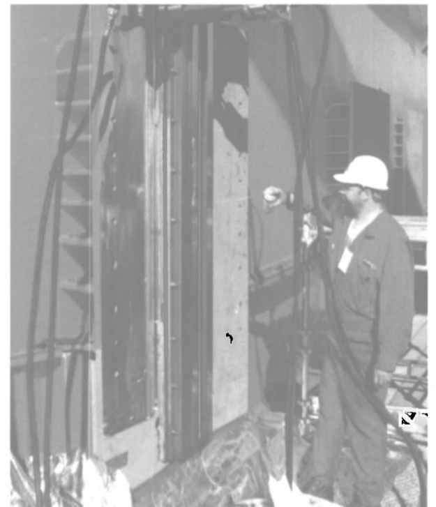
Above: A Norse Abandonment machinist lubricates the Climax PM6000 portable milling machine as it mills the steel plates on the Odin. A plate that has as much as 15 millimeters of steel milled from it is visible in the background.
