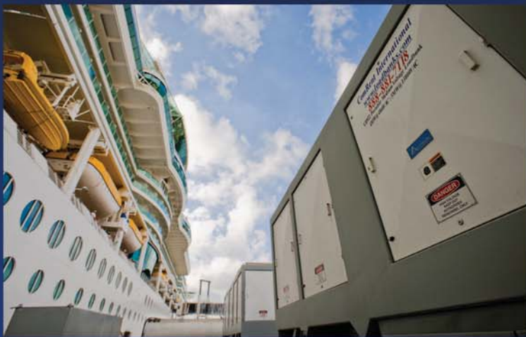
CR922 Medium Voltage Load Bank
