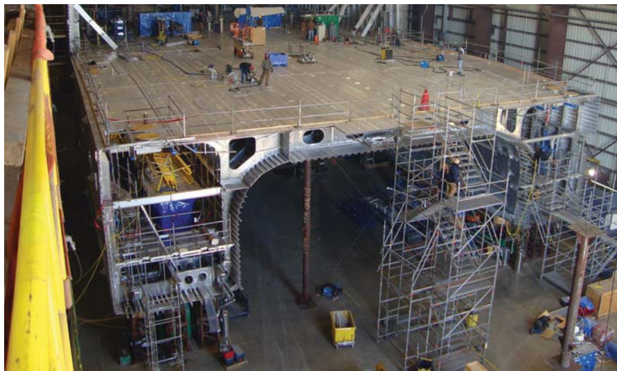
Taking Shape at Austal in Ala. is the USN's Joint High Speed Vessel (JHSV).
