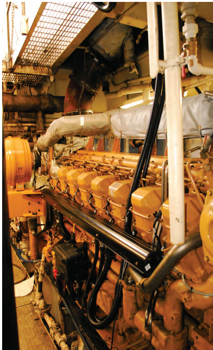
Caterpillar 3516B engine with 3500 emissions upgrade.
