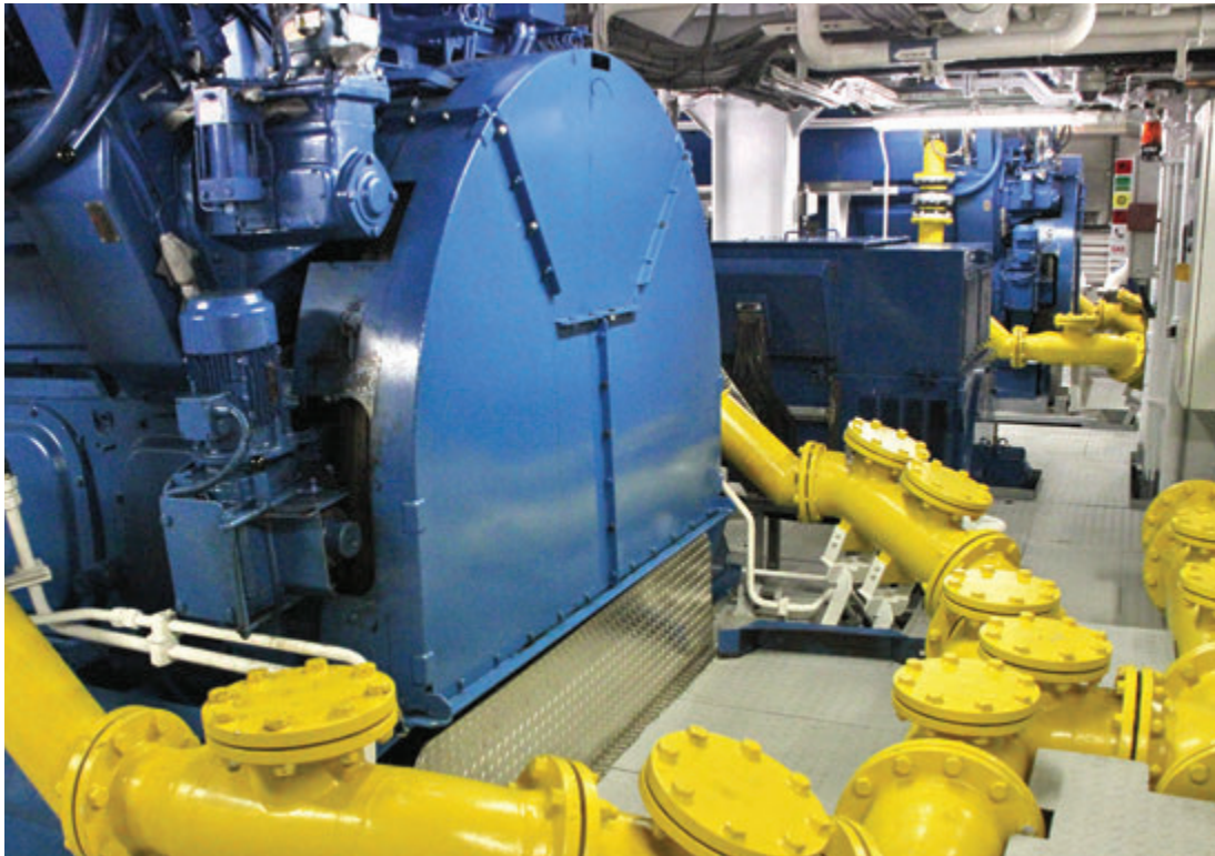
Above: The yellow painted double-walled pipes are indicating that they contain natural gas.
