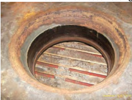
Picture 1: corroded housing
