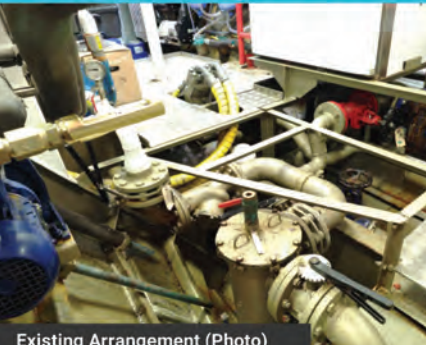
Existing Arrangement (Photo)
