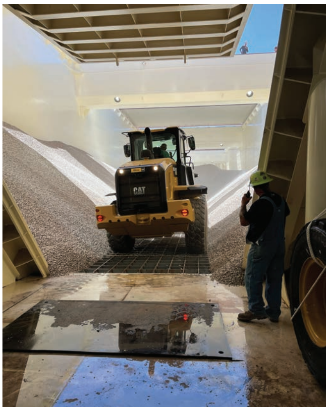
Figure 4. The vessel's cargo holds feature flat bottoms that accommodate the use of heavy machinery, which necessitated advanced coatings systems to protect these areas from damage.
