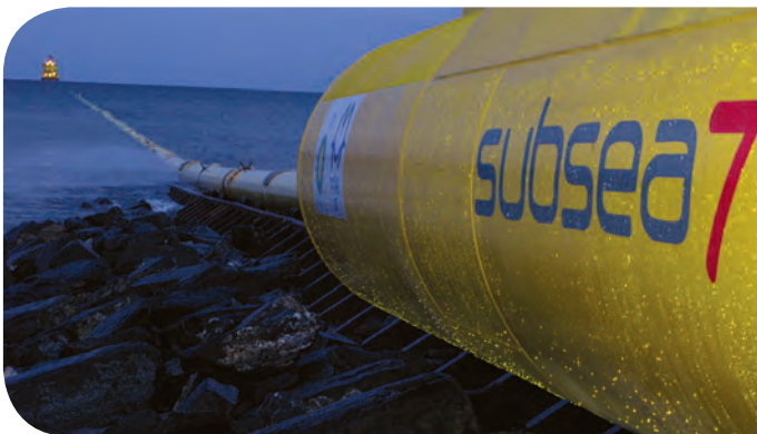
A vessel towing out a bundle, with the towhead in the foreground, at Wick, Scotland. Photo: Subsea 7.
