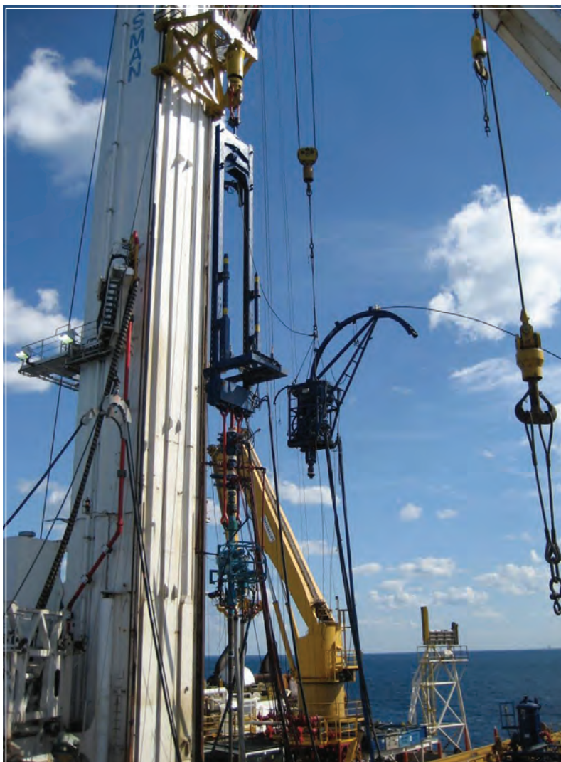
A crane atop the Q4000 rigging up coiled tubing to perform deepwater P&A work.
