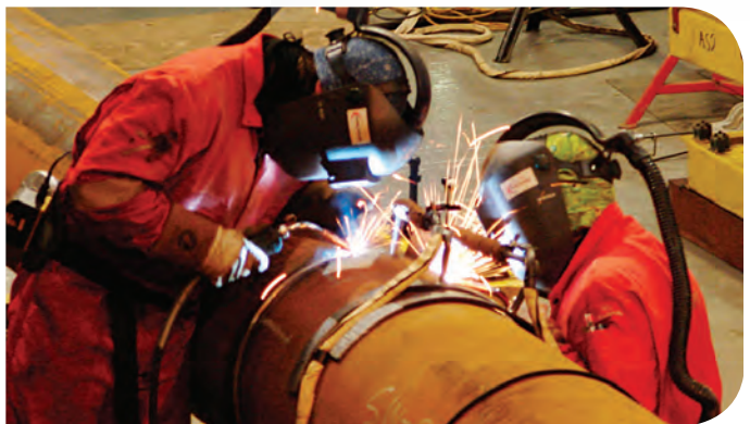
The firing line in fabrication hall's at the Wick facility. Photo: Subsea 7.
