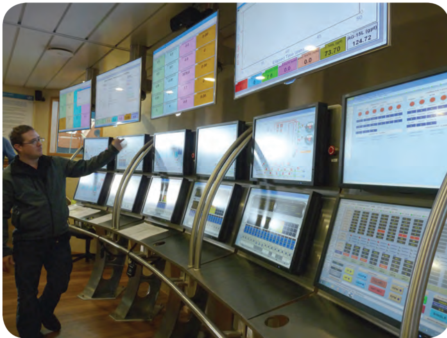
The Blue Orca's touch screen control room. Photo courtesy Elaine Maslin.
