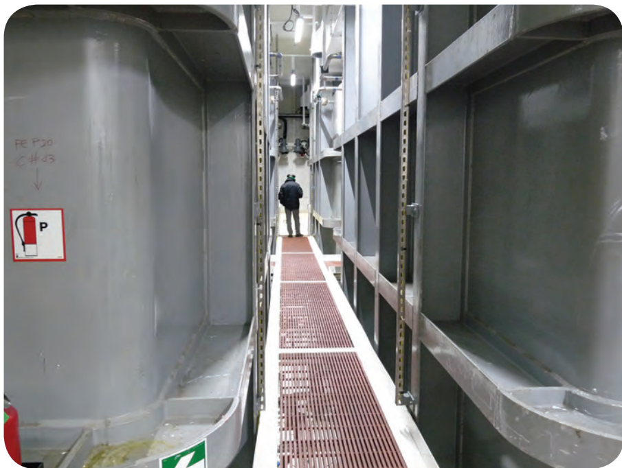
Enclosed tanks positioned above the main deck. Photo courtesy of Elaine Maslin.
