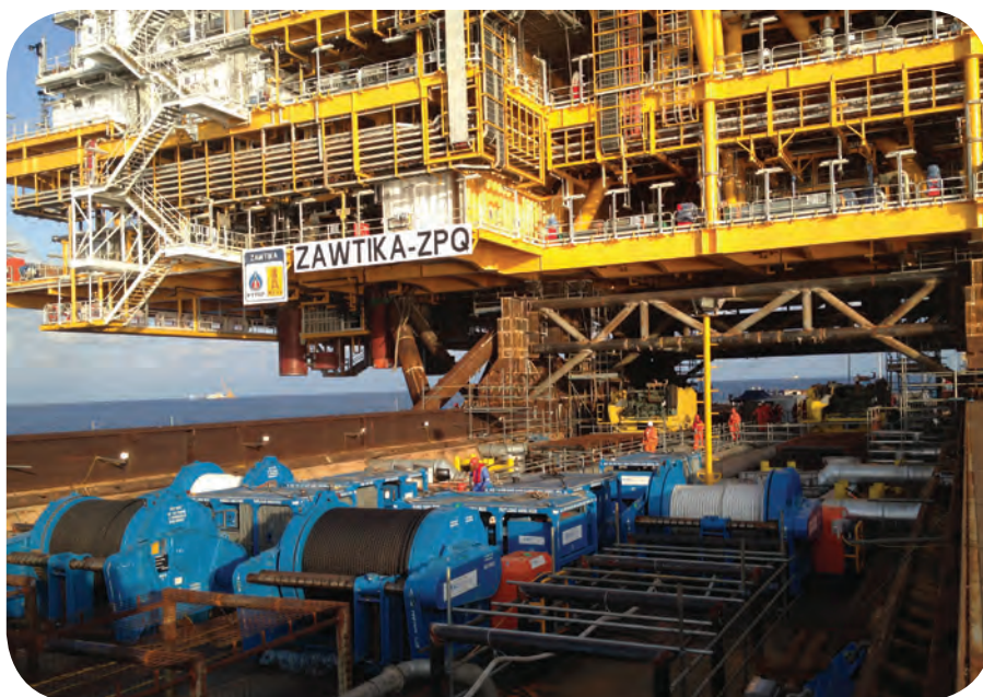
An ACE Winches floatover installation package on board the S45 Barge for work to install the ZPQ platform offshore Yangon, Myanmar. Photo from ACE Winches.
