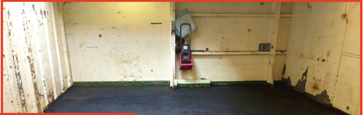
A container storage area was identified as suffering from severe corrosion or through wall defects totaling an area of 48sq m requiring repair.
