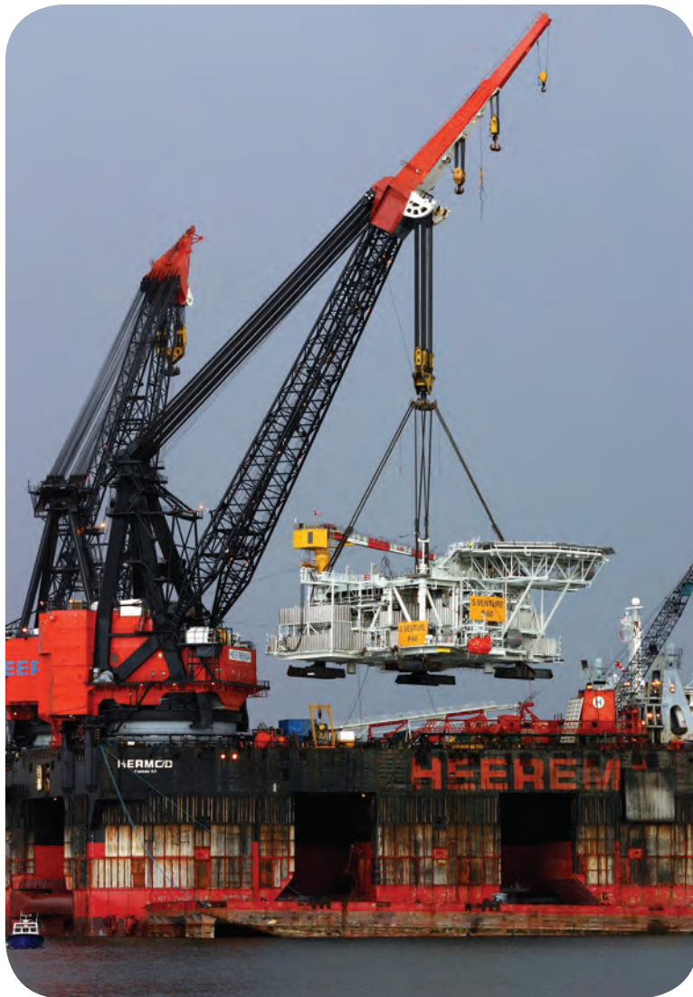
The Sable South Centre module being loaded ready for installation at the Sable Offshore Energy Tier II Compression Project, offshore Nova Scotia. Photo from Allseas.
