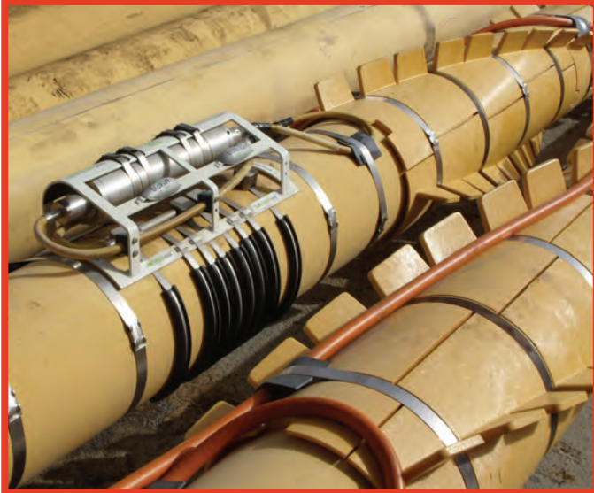
Motion loggers installed on a riser help assess fatigue.
