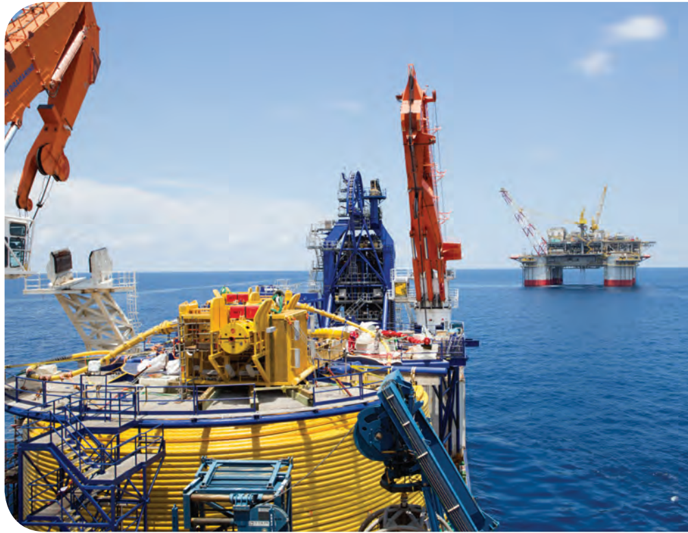
McDermott subsea construction vessel NO102 installed umbilicals totaling 65mi with other related subsea structures for Jack/St. Malo. Image from McDermott International.
