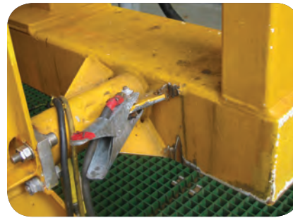
Damage from one of the guidewires to the lower cursor frame (LCF). The LCF sits in the moonpool area and acts as a guide/protection while deploying equipment through the moonpool and splash zone.
