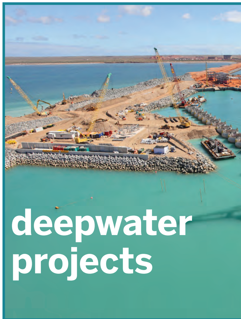
Engineers from Jumbo Maritime deliver 25 MOF caissons for the Chevron-operated Gorgon development offshore Western Australia, in 2012. Photo from Jumbo Maritime.
