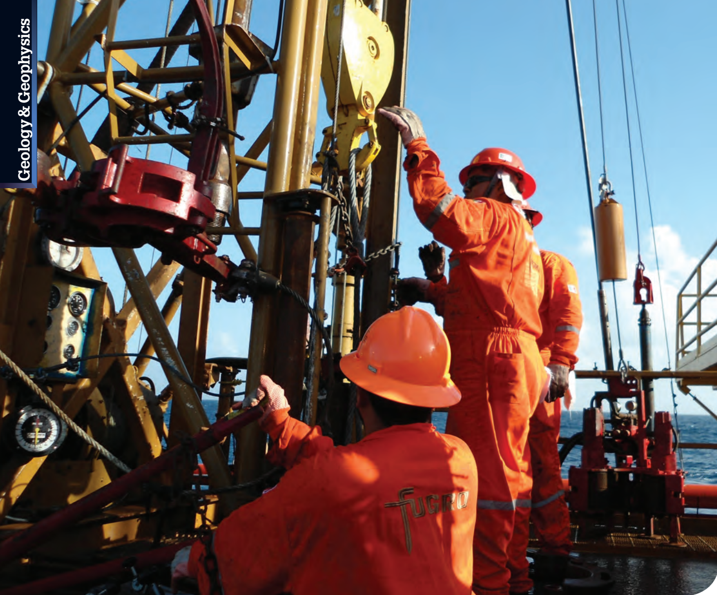
Acquiring geotechnical data for platform foundation design in Mexico's Bay of Campeche
