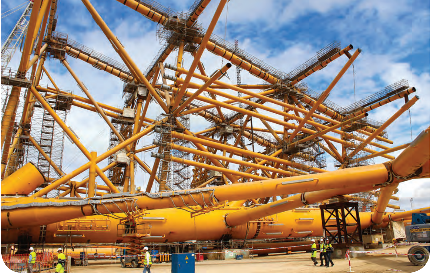
The 22,400-tonne Mariner jacket under construction at Dragados Offshore's yard in Cadiz, Spain.
